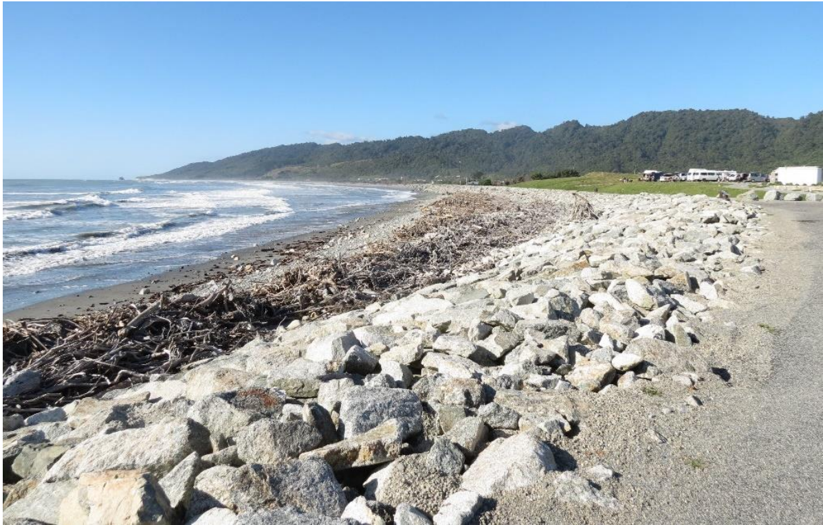
Figure A-5: Accumulating beach and driftwood debris in front of the new dumpsite revetment. An access track separates the revetment from the grassy dumpsite area (at right). Date: 05-03-2020 [Credit: M. Allis (NIWA)].
