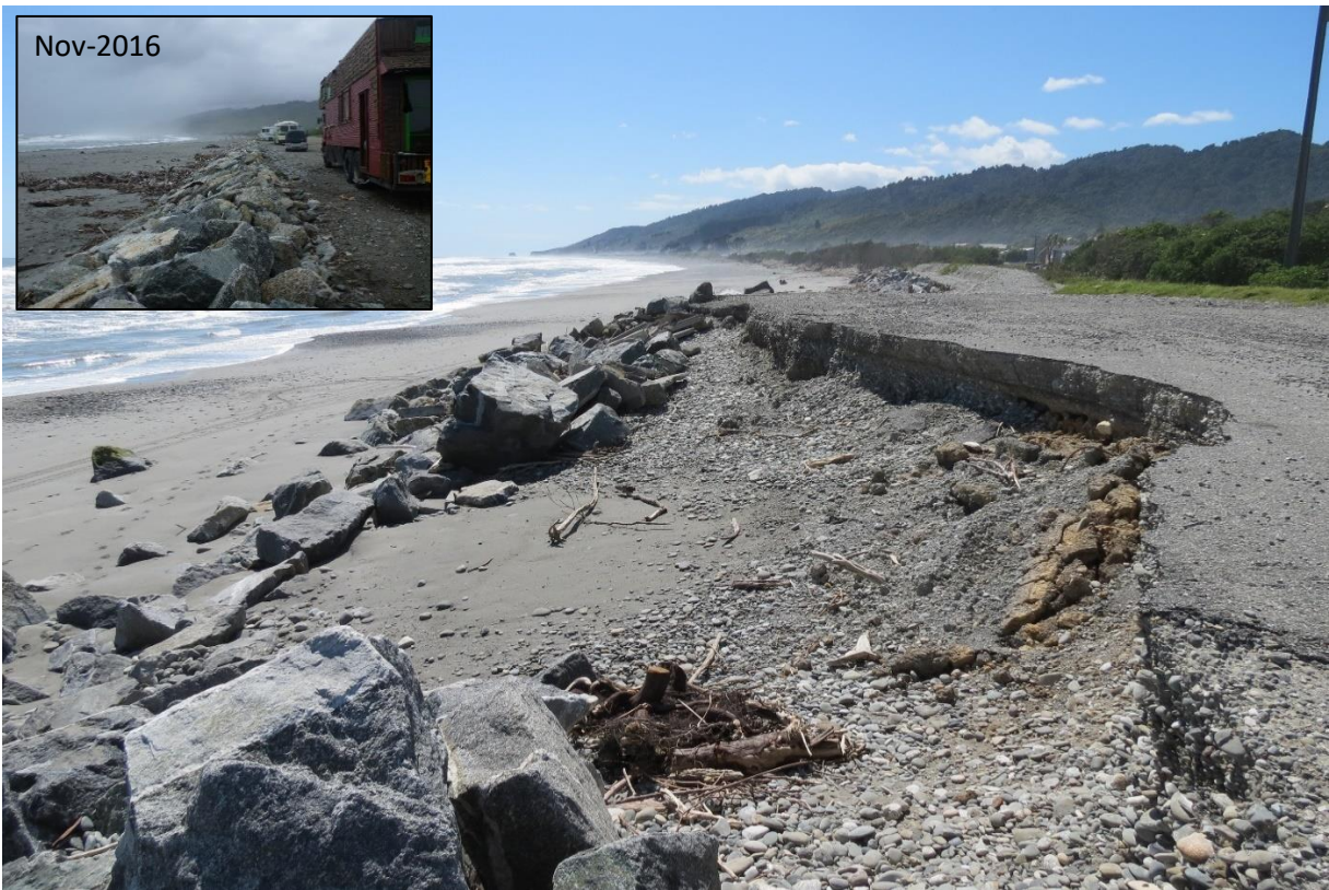
Figure 2-2: Erosion and undermining of carpark in 2020 and the same view in 2016 (inset) The elevation of the beach reduced by 2-3 m [Dates: 05-03-2020, 21-11-2016 (inset). Credit: M. Allis, M. Hicks (inset) ].
