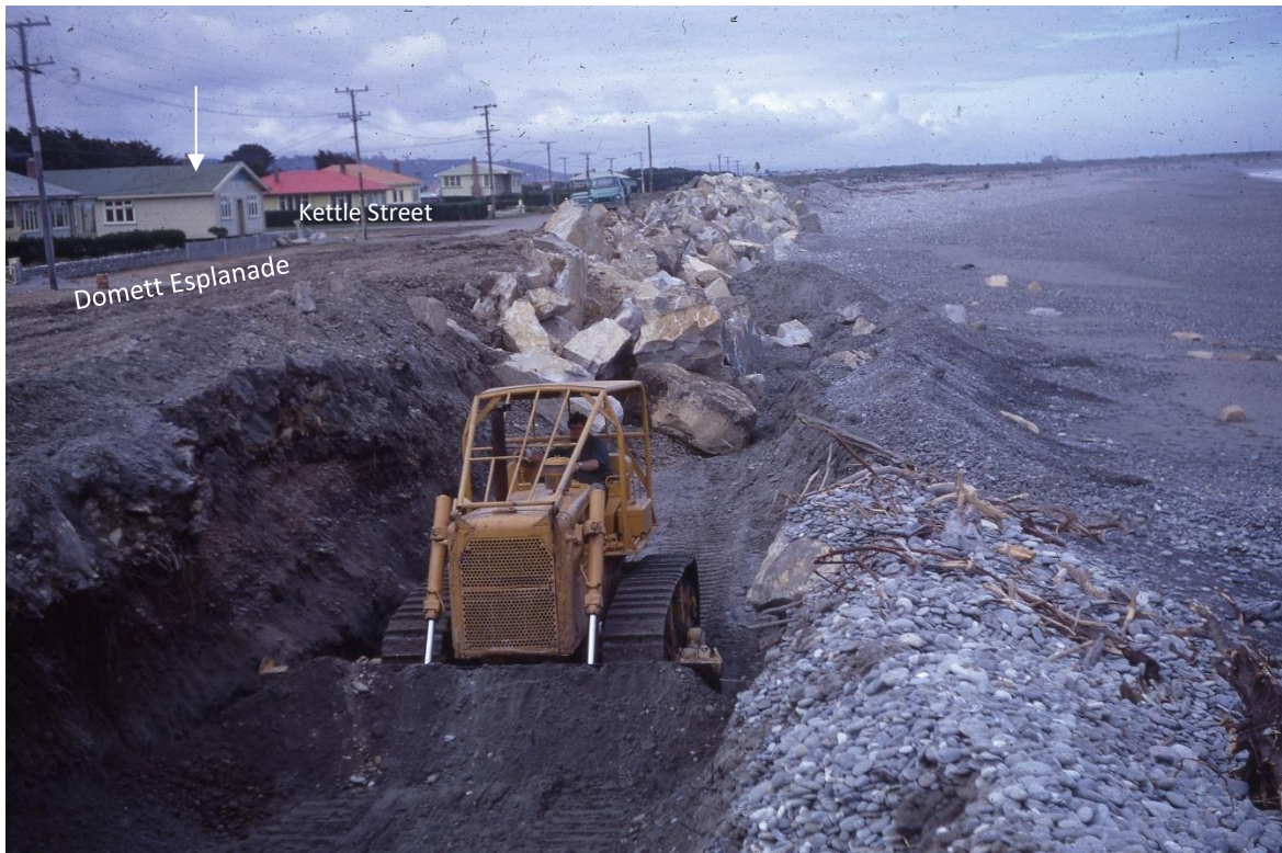
Figure 2-5: 1969 photograph of Cobden rock wall under construction. View south towards Greymouth. No. 90 Domett Esplanade indicated with arrow. [Source: pers. comm. Paulette Birchfield].
