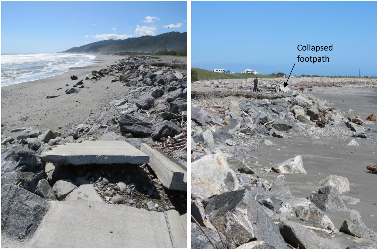
Figure A-1: Collapse of upgraded carpark features at Cobden Beach. View to south (left) and to north (right). Arrow (right) shows collapsed concrete footpath and kerb from left photo. Man and dog for scale (right). Date: 05-03-2020. [Credit: M. Allis (NIWA)].
