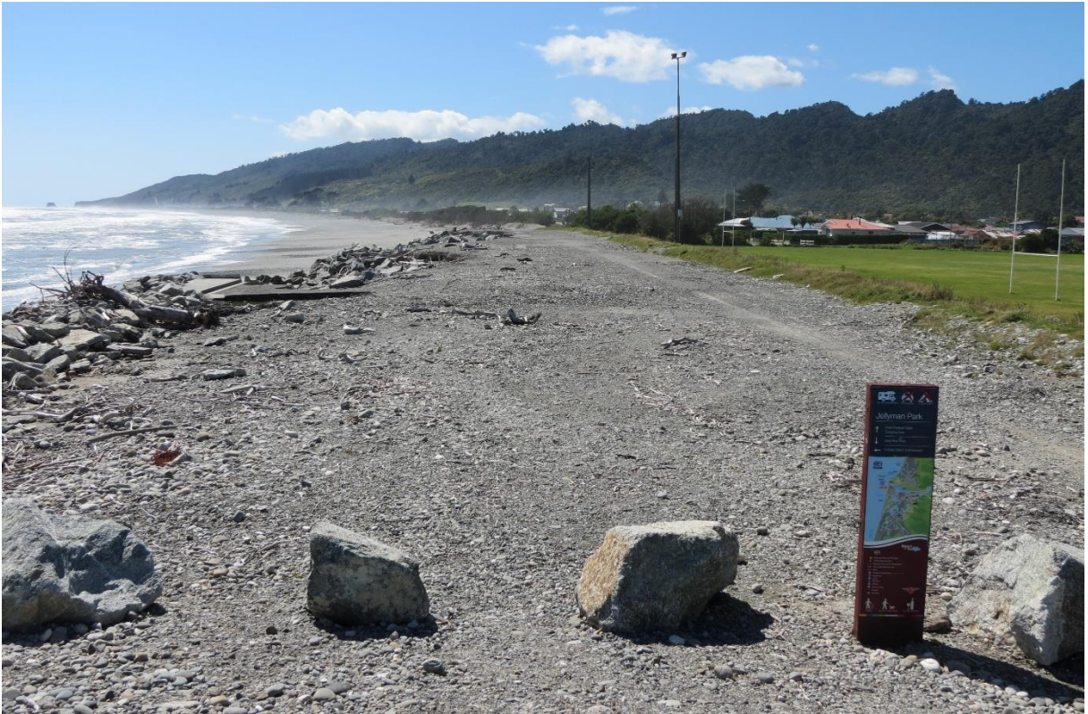
Figure 2-3: Eroded carpark and revetment between Cobden Beach and Jellyman Park. Date: 05-03-2020 [ Credit: M. Allis (NIWA) ].
